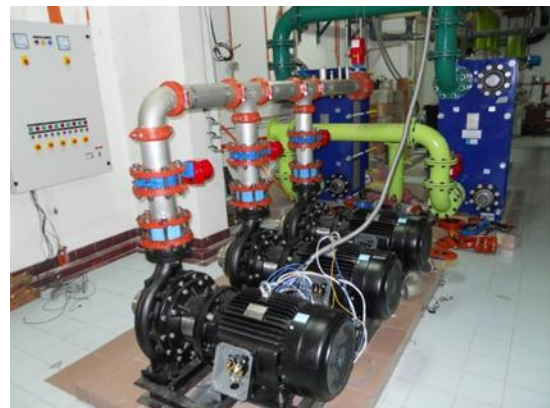
FIG. 3. New primary pump.
